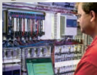
Priority One® consolidates and integrates all facets of the production line into one comprehensive control operating system.
